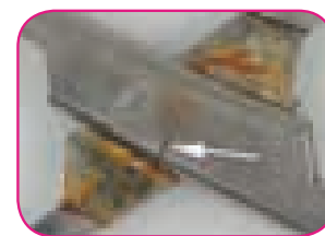
Box joint showing cracking & biological debris
